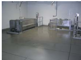
SlipNOT® stainless steel flooring in a cheese processing plant.
